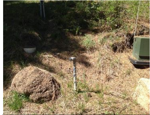
One of the 18 water risers located throughout the community.
